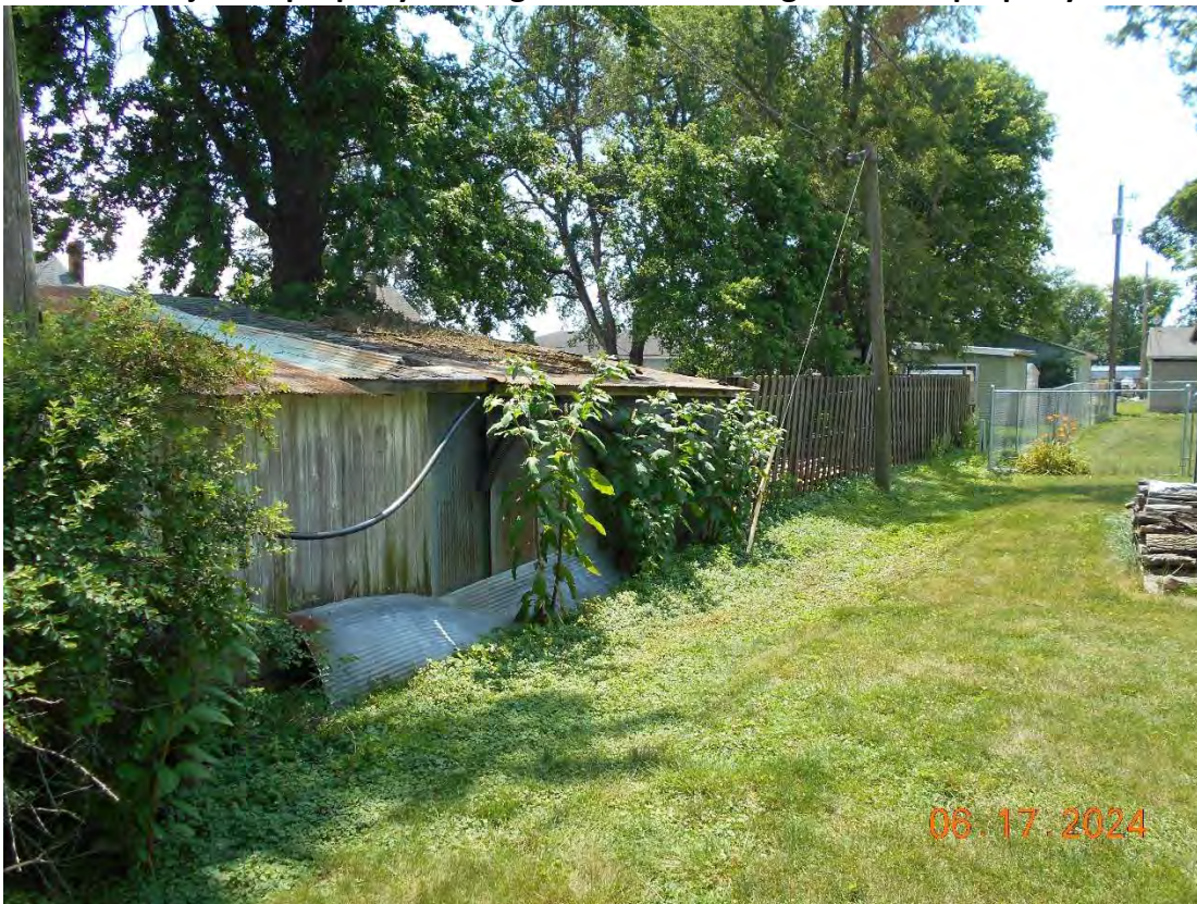
From adjacent property looking SW toward existing shed on N property line
