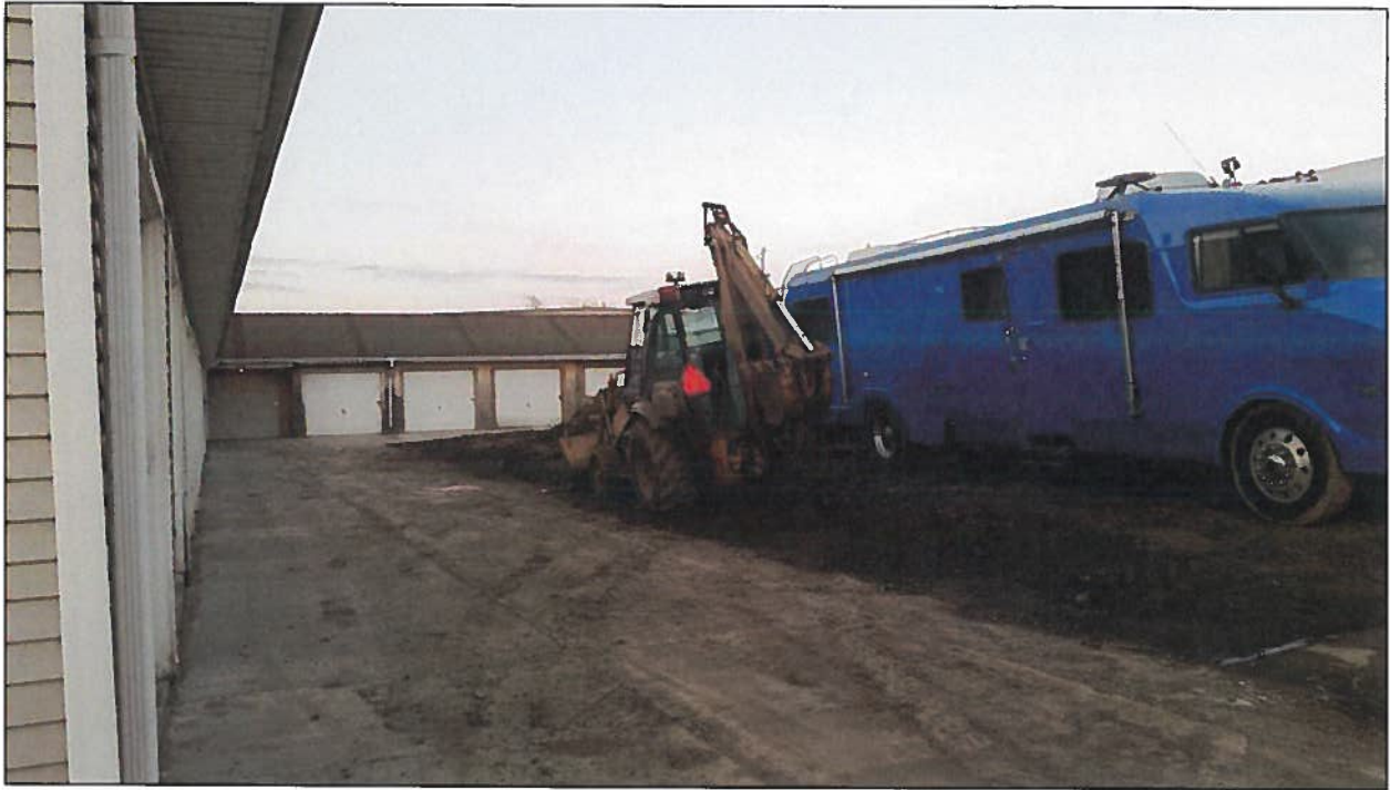
Center storage area to east of bus maintenance area, facing north from driveway
