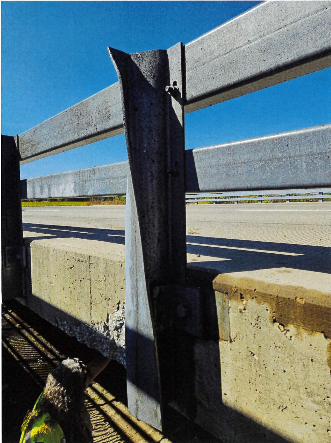
Post two twisted, and spall visible
