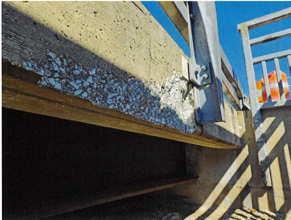
Post two – spall
